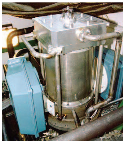
Fig 6 Turbo-generator as assembled to the ORC power plant
